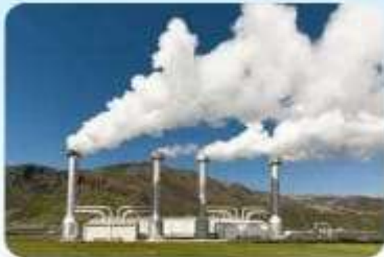
Geo thermal power plant
